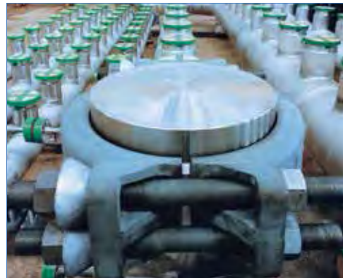
Test and production manifolds
